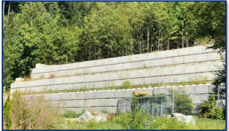
Unattractive visually dominant retaining wall.
