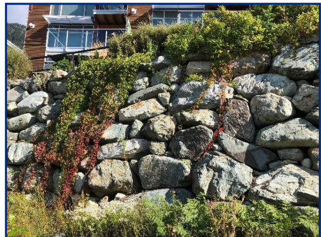
Retaining wall is made with natural building materials and visual impact is minimized with natural landscaping.
